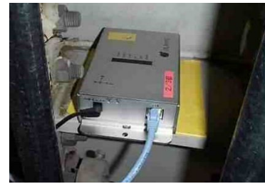
(a) ITK-002 for Hazawa Tower
