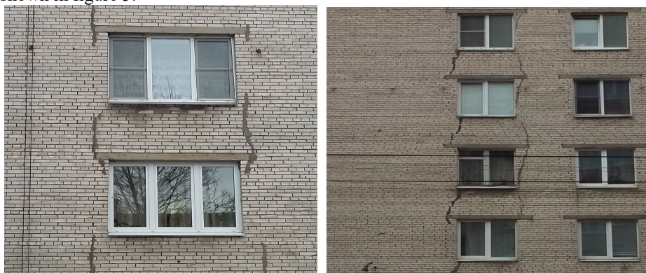
Fig. 4. The significant cracks appearance in the surveyed administrative building
