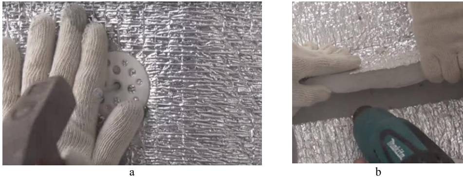
Fig. 1. Installation of thermal insulation: a – mechanical fixation of the insulator sheet; b – welding of joints of the polyethylene foam rolls.
