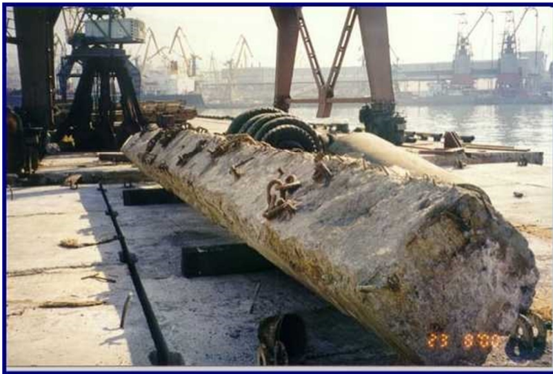
Fig. 2. Edge beam before the repair.
