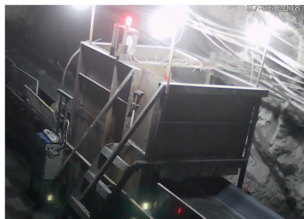
Fig. 6. OCS RLP-21T on the main conveyor of the NPR.
