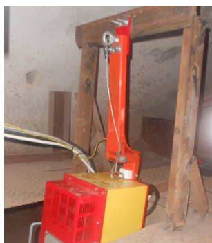
Fig. 7. OCS RLP-3-02 on conveyor No. 1 at ZPP-1.
