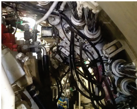
Fig. 7. Active laser target inside the shield. (Tashkent-2018).
