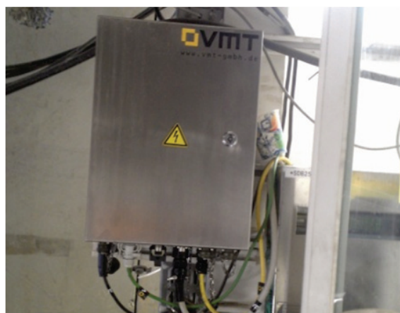
Fig. 9. Central Radio Modem (Switch). (Tashkent-2018).
