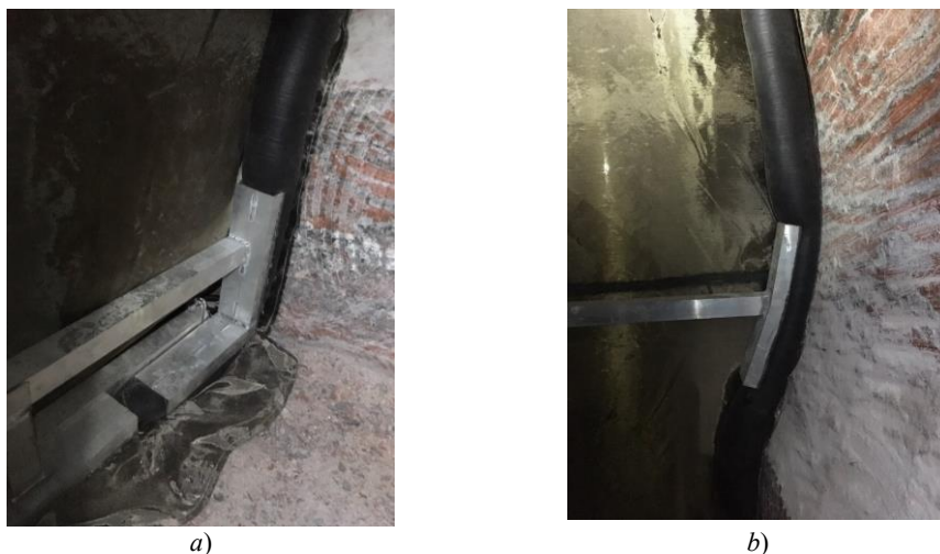
Fig. 3. Pressing the air hose: a – against the soil; b – against the wall of the mine opening
