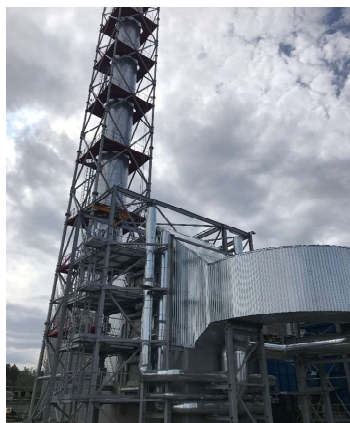
Fig. 2. The flue condensing economizer (CE) recently installed at CHP-6
