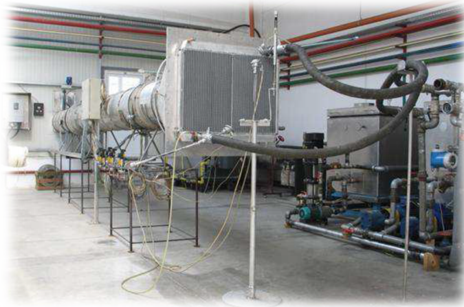
Fig. 2. Thermal and hydraulic performance test bench at RAAL S. A.
