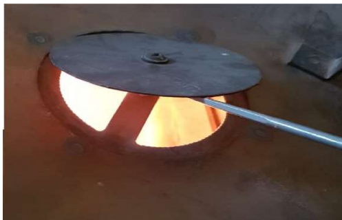
Fig.4 Aspect of flame inside the boiler furnace
