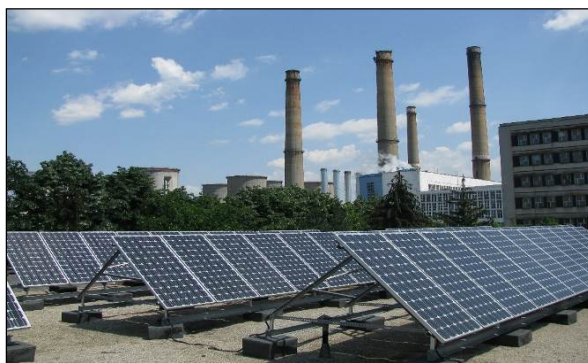
Fig. 1. Photovoltaic installation with installed power - 22kWp - INCIDE ICEMENERG [15]
