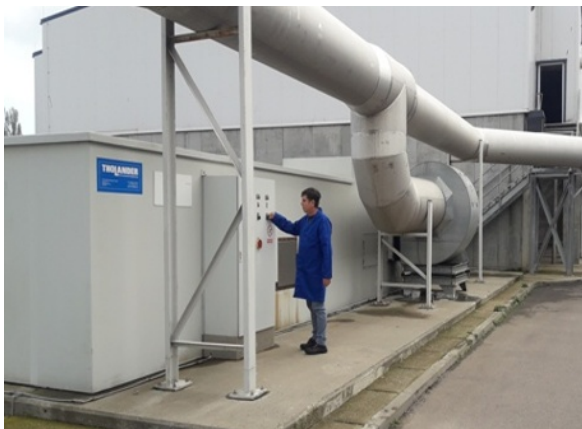
Fig. 6. Deodorized air defective station mechanical cleaning stage
