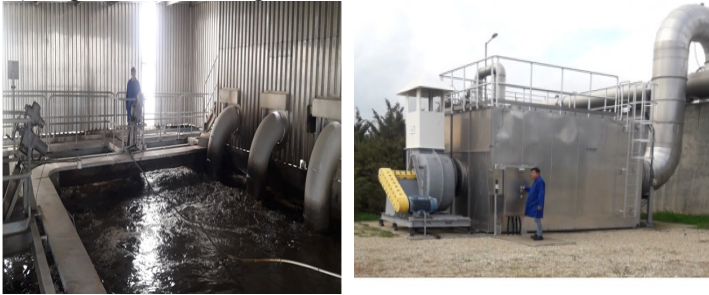
Fig. 5. View of the bioreactor distribution chamber
