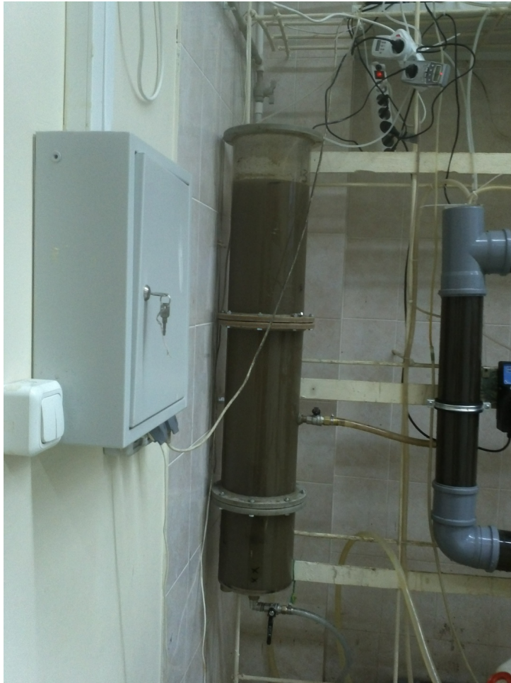
Fig. 2. A photo of the Sequencing Batch Reactor plant.
