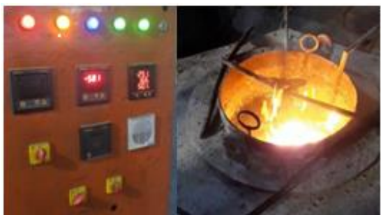
Fig. 3. Digital temperature indicator and Controller
