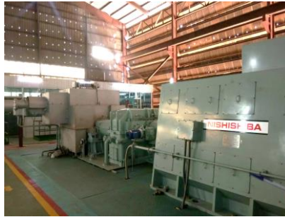
Fig. 5. Steam turbine-generator brand SHINKO with 9 MW capacities.
