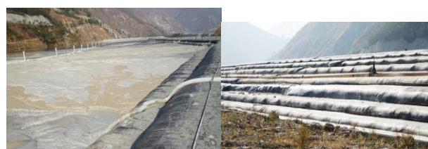
(a) Inside of tailings dam (b) Outside of tailings dam Fig.1 Close-in partial view of tailings dam using geofabriform method in Yunnan province
