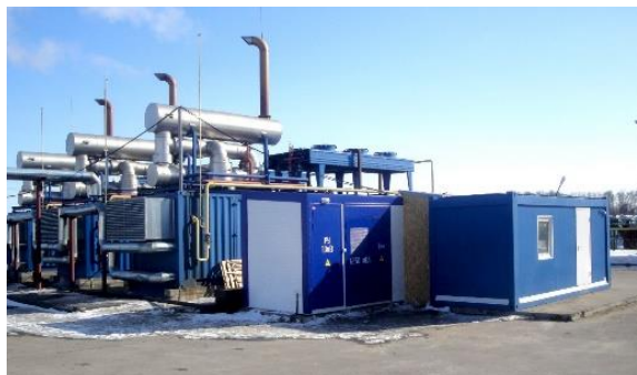
Fig. 1. Experimental power system for testing the combined work of ESS-10-1200-400 and GEG.
