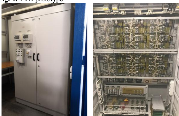
Fig. 5. Thyristor switch cabinet.
