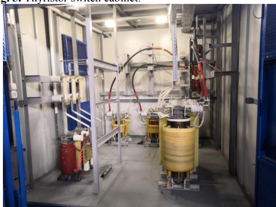
Fig. 6. Power transformer compartment.
