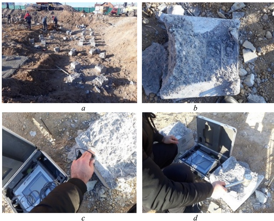
Fig. 1. Measurement process (driven piles): a – pile field; b – pile surface; c – sensor installation; d – blow produc
