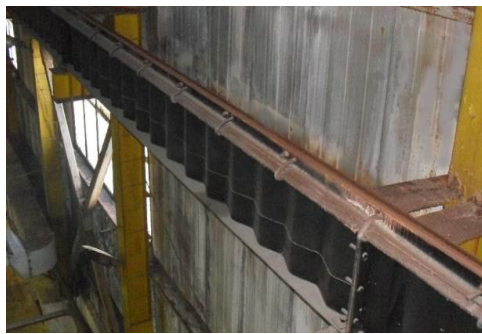
Fig. 6. Crane beams in the main building of the plant in Almaty region. The height of the beams is 640 mm, the thickness of the corrugated walls is 6 mm. 2001.
