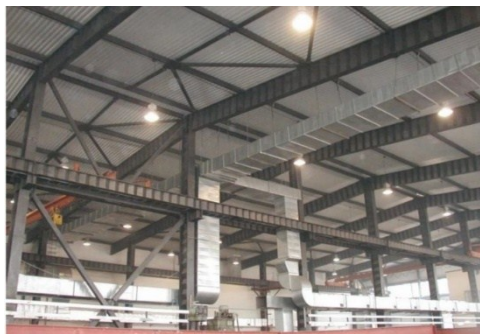
Fig. 5. One-story steel frame of the industrial building, in which the roof girders, columns and crane beams are made of welded I-beams with corrugated walls. Seismicity 10 points. 2007.
