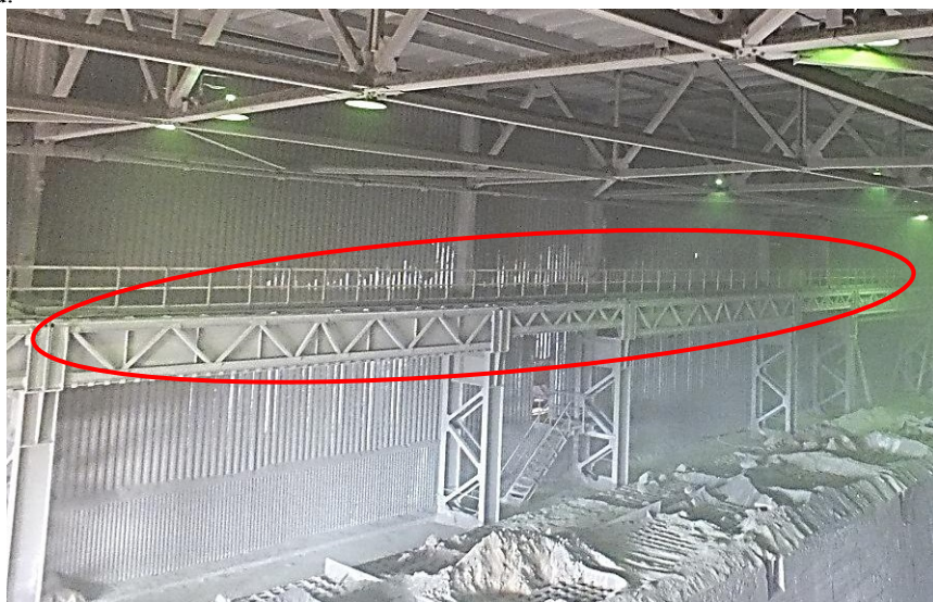
Fig. 8. General view of reinforced steel crane beams along the A axis with spans of 12 and 6 m.
