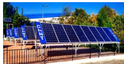
Fig.1. Solar photovoltaic station with capacity of 10 kW connected to low voltage network of the Faculty of Power Engineering
