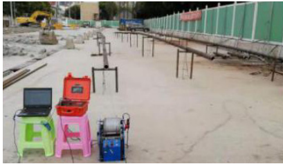
Fig.2 Horizontal fiber optic gyroscope inclinometer test
