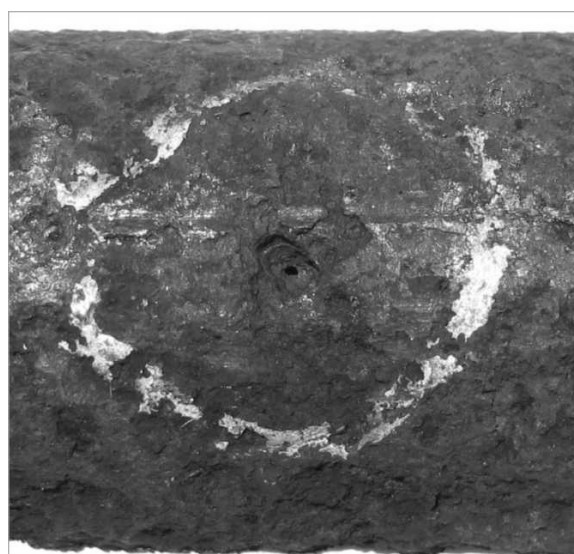
Fig. 6. The nature of the corrosion damage to the tube.
