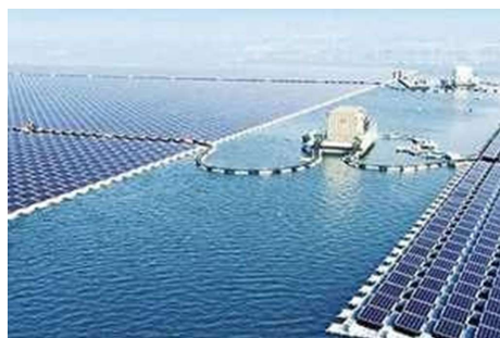
Fig.2. A floating photovoltaic plant on an artificial lake in Anhui Province in China
