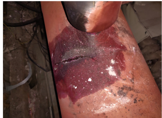
Fig6. Circumferential cracking of the base material of heating and desuperheating pressure reducer pipe.
