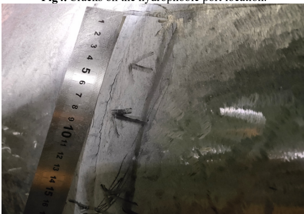
Fig5. Cracks on weld fusion line of the high voltage bypass desuperheater pipe.
