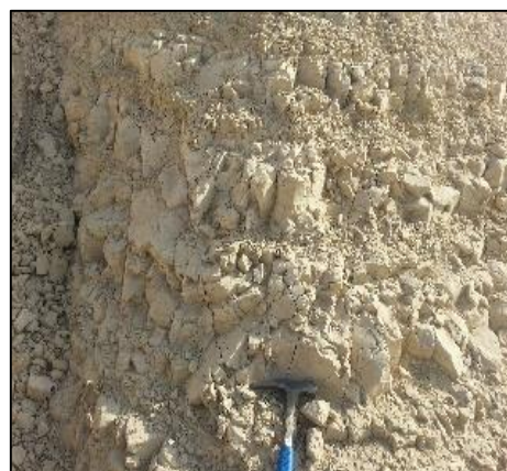
Fig. 11. Limestone layers dipping slightly to the South and highly fractured (Source: Field survey, 2017). Hammer for scale.
