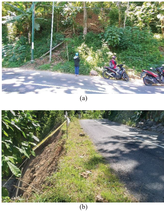
Fig. 2. The landslide occurred on the main road from the east of Samigaluh District: (a) on the right side and (b) on the left side.
