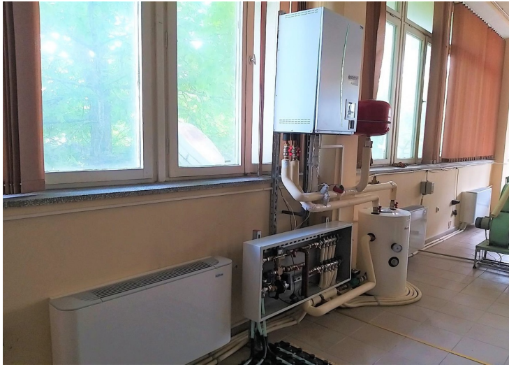
Fig. 2. General view of the AWHP system.
