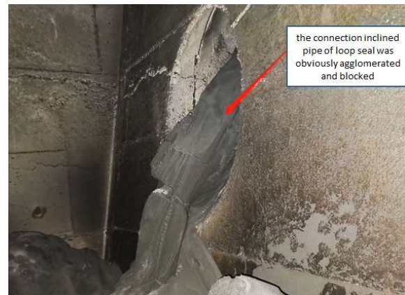
Figure 3. The blockage of loop seal
