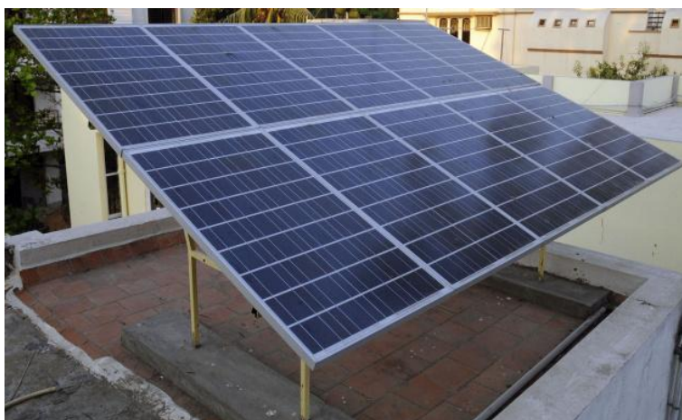
Figure 9: Roof top Solar Power heater and plant
