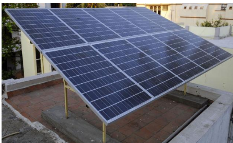
Figure 9: Roof top Solar Power heater and plant
