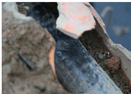
Fig. 2. Outer sheath depression
