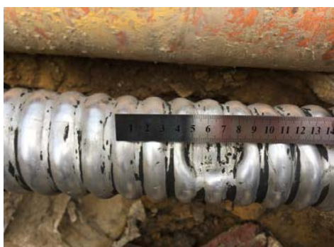
Fig. 3. Damaged aluminum sheath
