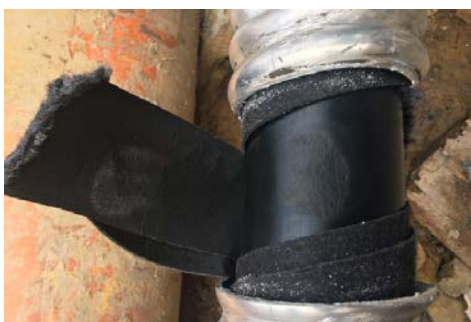
Fig. 4. Damaged insulation shield
