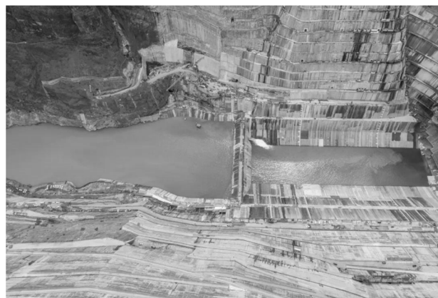
Fig.4 Effect diagram of the first water filling process in the cushion pool of the project
