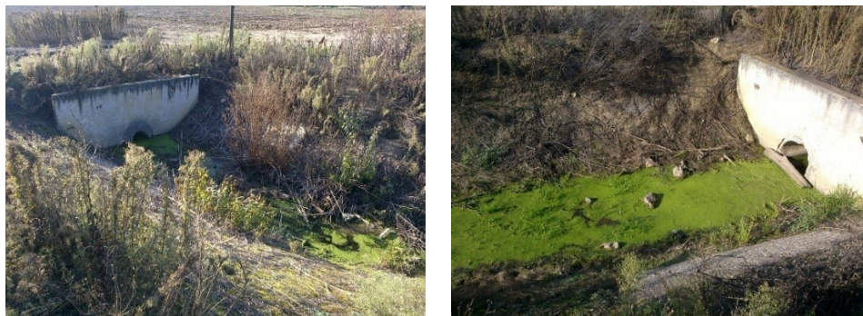
Fig. 1. Condition of the drainage canal and its facilities in long-term operation without current and capital repairs
