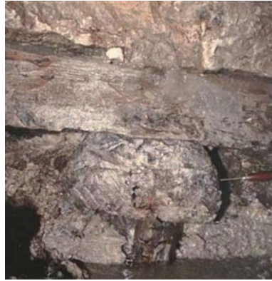
Fig. 3. Biological deterioration of a log house. Kostroma Region.
