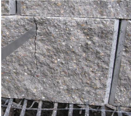
Fig. 11. Fragment of the MSE-wall lining with a defect
