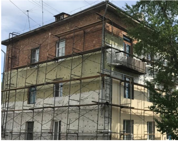
Fig. 6. Defects in the installation of hinged facade systems
