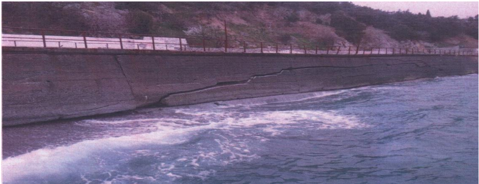
Fig. 1. Emergency condition of coastal protection structures in Yalta (Simeiz)
