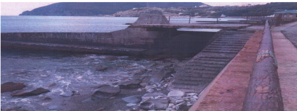
Fig. 2. Emergency condition of coastal protection structures in Yalta.
