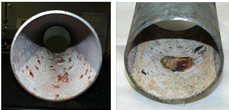
Fig. 2. Photograph showing tubercles and pinhole (circled) leakage of galvanized steel sprinkler pipe in dry pipe systems [8].
