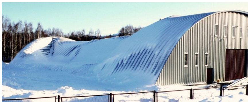
Fig. 2. The example of the collapse of a frameless arched building
