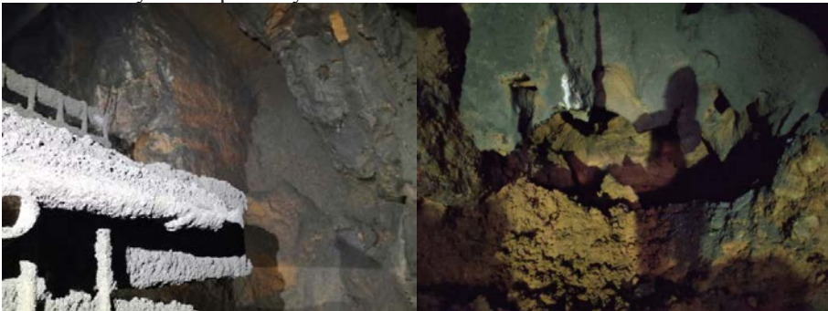
(a) Karst caves on the right wall of the entrance of Xinjie Tunnel YK48+080 mileage (b) Karst cave on the left side of Xinjie Tunnel ZK50+837 mileage
