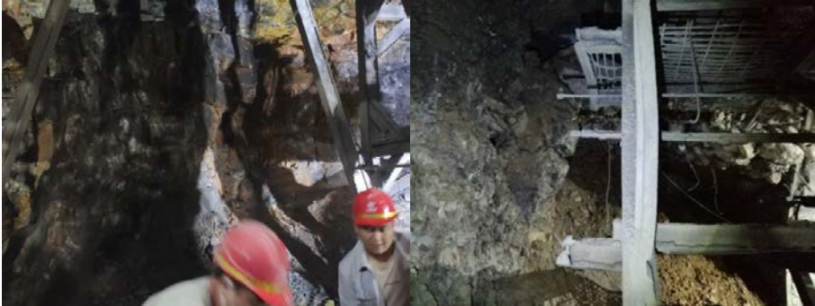
(a) Xinjie Tunnel YK49+580 mileage central karst cave (b) The karst cave on the right side of the tunnel face ZK48+389 mileage of Xinjie Tunnel
