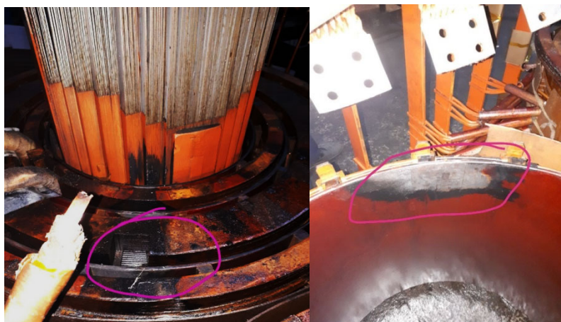
Fig. 5. Fault detected in traction transformers.
