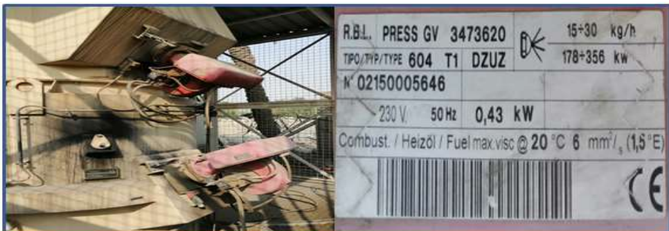
Fig. 3 Characteristics of the burner used in the two combustion chambers
