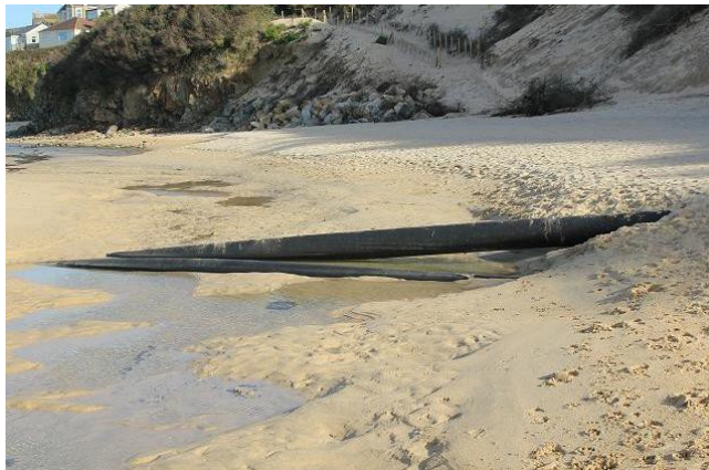
Fig. 11 Cable unearthed under the action of waves [6]
