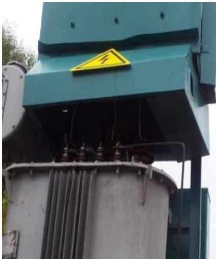
Fig. 1. Photo of the transformer housing installed at the 6-10 / 0.4 kV mast-type UTS of the branch of “IGDC of the Center” – “Orelenergo”.
