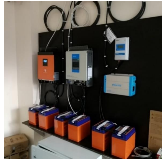
Fig. 2. General view of the auxiliary equipment of the experimental array
