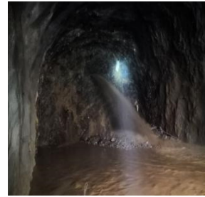
Fig. 4. Water gushes out of the excavation face
