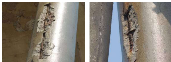
Figure 2. exposed corrosion of steel bar
