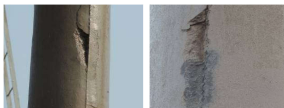
Figure 3. Concrete protective layer bulges, cracks and falls off
