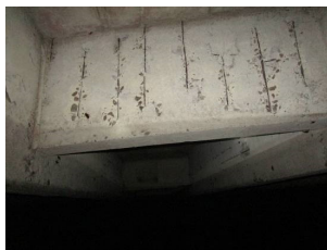
Figure 4. Exposed reinforcement of diaphragm plate.
