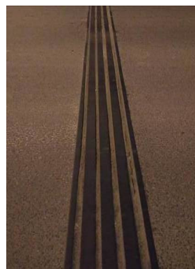
(b) Modular expansion joint (Mingzhou Bridge)
